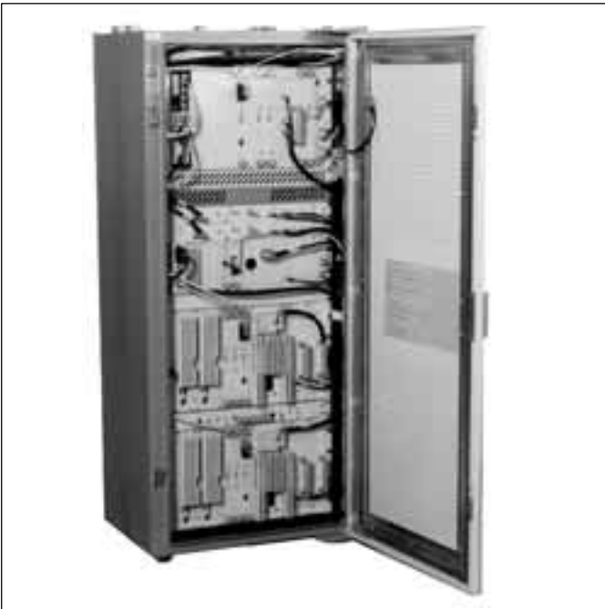
Base station of cellular network
